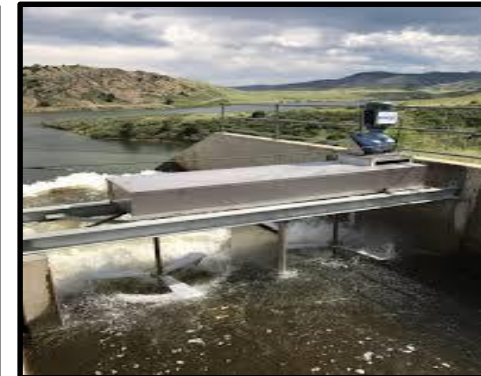
Emrgy River Power Plant
