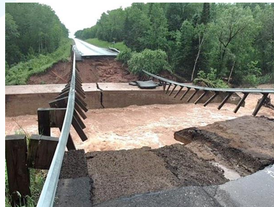
2018 Flooding HWY 2 WI
