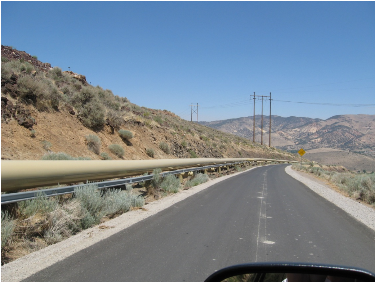
Photo 2: Typical Insulated Geothermal Pipeline with Electrical Cables
