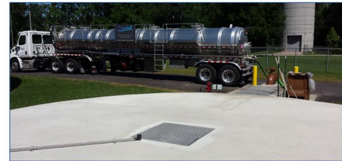
Photo 3: High strength equalization tank with truck, Waste Water Treatment Facility, Stevens Point, WI
