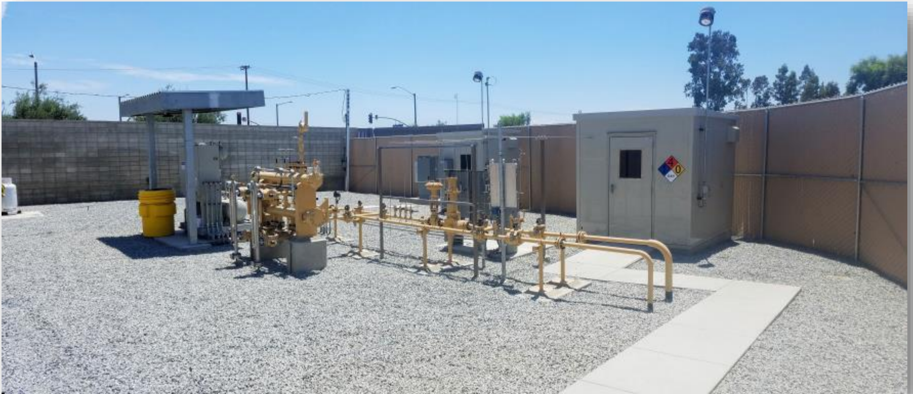
SoCalGas Pipeline Interconnect- Point of Receipt
